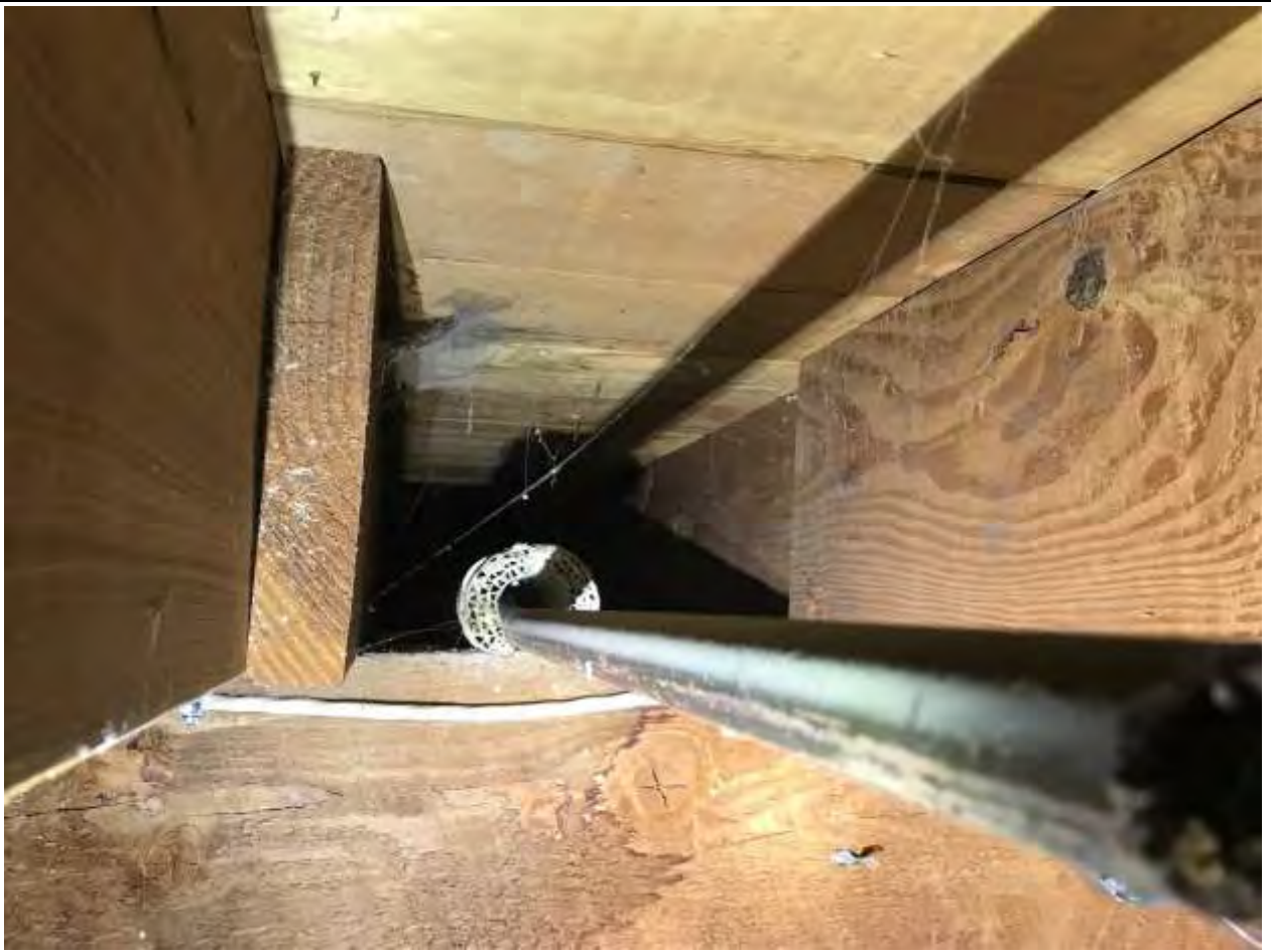
Picture No. 5: Corrugated asbestos paper on redundant piping in the crawlspace
