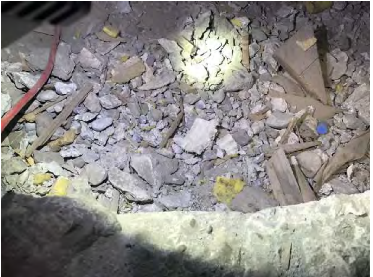
Picture No. 8: Asbestos paper pipe insulation debris within crawlspace dirt
