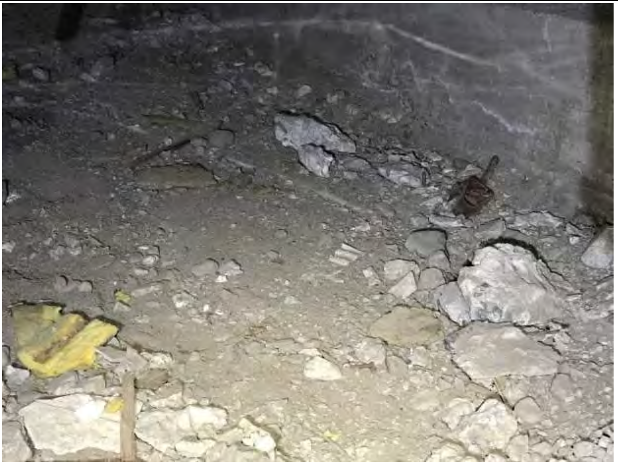
Picture No. 7: Asbestos paper pipe insulation debris within crawlspace dirt
