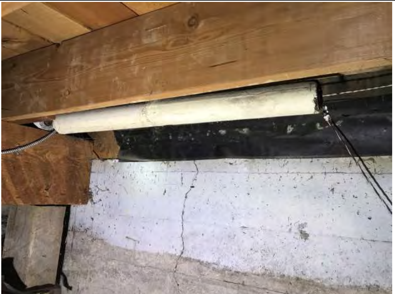
Picture No. 6: Section of redundant corrugated paper asbestos paper pipe insulation
