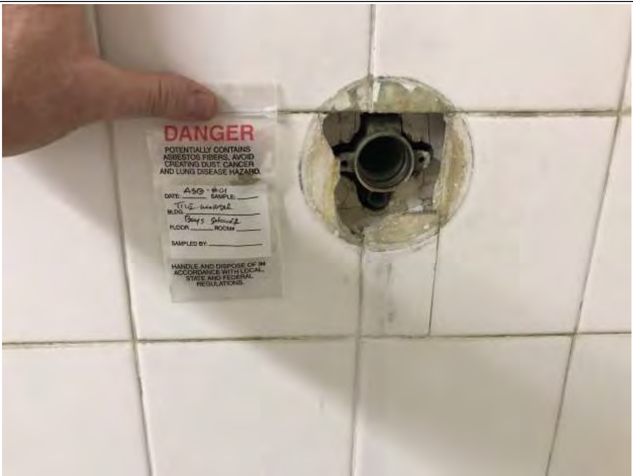
Picture No. 3: Sample 1 of mortar for asbestos content – results indicate no asbestos was present in the tested mortar
